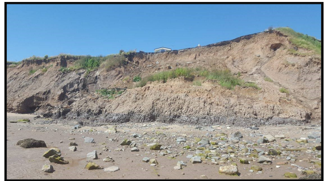
Figure 6: Evidence of erosion and unstable cliffs with processes such as slumping visible.
